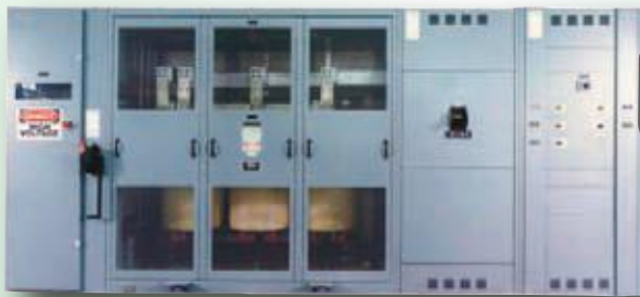
Indoor Unit Substation
