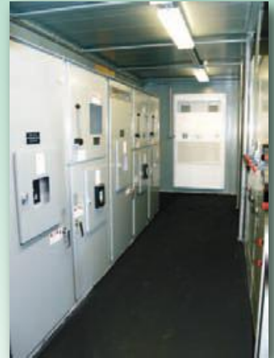
Outdoor Walk-In Metal Clad Switchgear
