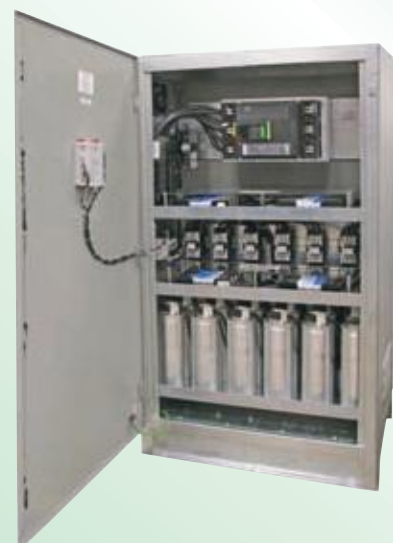
Figure 2 : Power Factor Improvement (PFI) Plant
